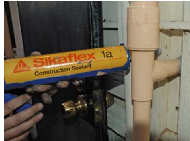
Exposed PVC pipe is painted to protect it from UV degradation. The hole is sealed with an adhesive sealant to prevent moisture from entering.
