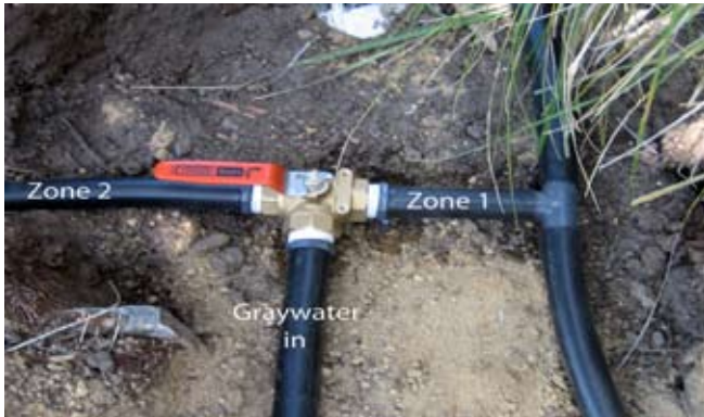
This 3-way valve creates two zones in the landscape. Water can be redirected from one zone to another zone by turning the handle. Photo: Laura Allen.
