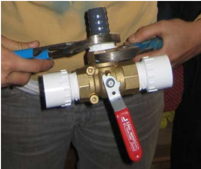
Tightening fittings onto the 3-way valve with channel locks. Photo: Laura Allen.
