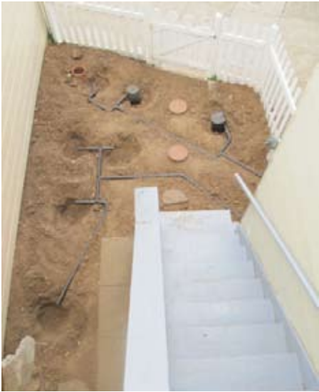
Sample image of a graywater system pre-burial. Photo: Josh Lowe.
